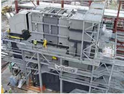
The Balcas plant near Enniskillen in County Fermanagh, Northern Ireland, makes wood pellets from sawdust and woodchips, with a capacity of around 50,000 tonnes per year. Balcas chose to invest in the plant after a 40% increase in business had led to a surplus of sawdust and woodchips at their timber-processing plant. Its energy supply is provided by biomass-fuelled CHP (11.5MWth/2.7MWe) VYNCKE
